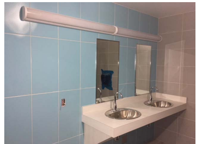
Finishing Work – Sinks, faucets, mirrors and lighting has been installed in washrooms and change rooms.
