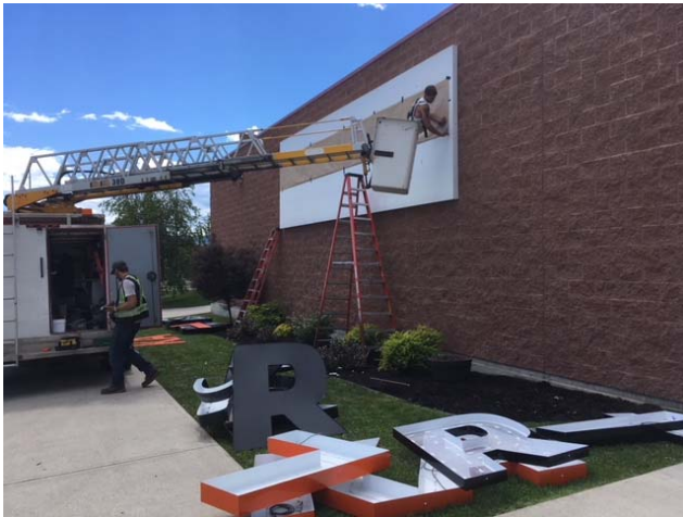
Signage – New updated signage is installed on the existing Kal Tire Place.
