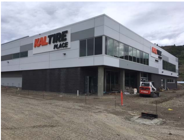
Signage – The two new Kal Tire Place North signs are installed on the east and north sides of the rink.
