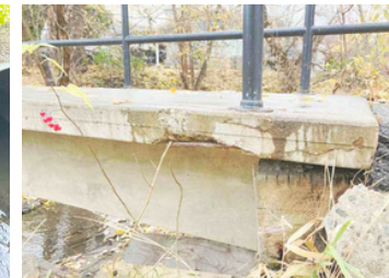
FULL DEPTH CONCRETE SPALL AT DECK SOUTHEAST CORNER
