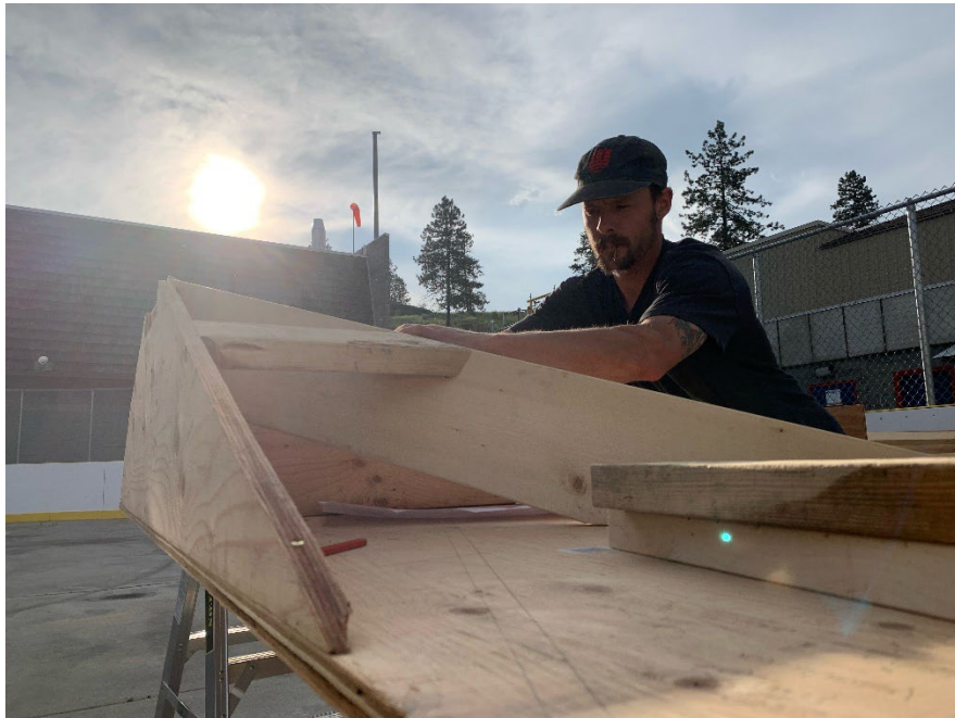
Above: Seamus Townsend builds a ramp for the temporary indoor skatepark at the Vernon Curling Club.
