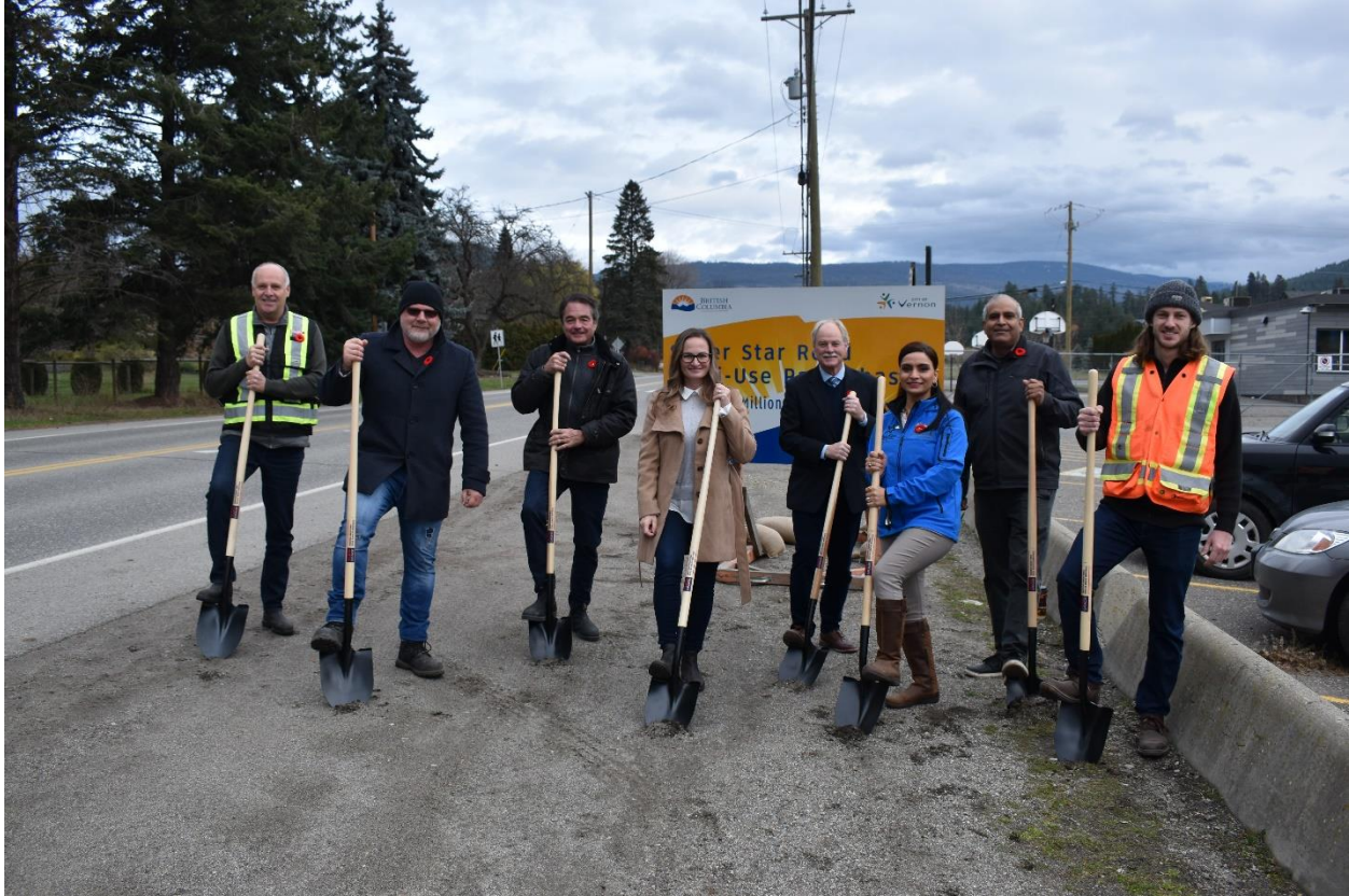
Ground is broken for a new multi-use path between Pleasant Valley Road and Blackcomb Way. (Pictured above L-R: Coun. Brian Quiring, Coun. Kelly Fehr, Coun. Scott Anderson, Coun. Kari Gares, Mayor Victor Cumming, MLA Harwinder Sandhu, Coun. Akbal Mund, Jordan Peterson, Project Engineer, Stantec.)
