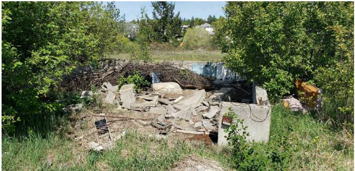
Photo 4 Building foundation and debris (to be removed) along west boundary of the Site. Aspect north.
