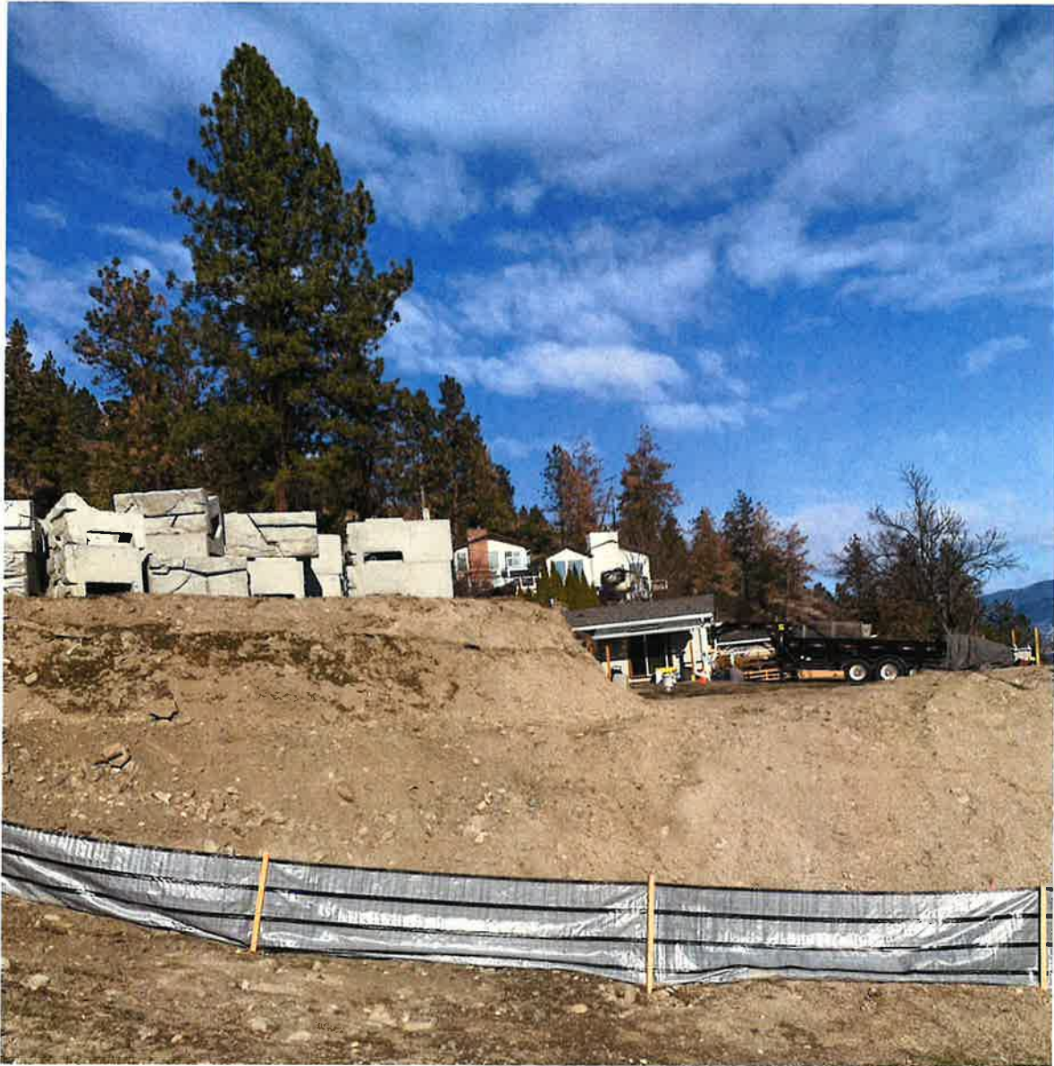
Photo 1: Verti-blocks, site fill and grading and silt fencing (approx. location of retaining wall)
