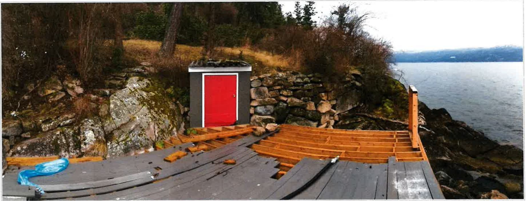
Photo 2. Close-up of HWM / SB, SPEA vegetation, pump house and deck to be removed (from proposed dock area - looking SW) – Dec. 14, 2020.
