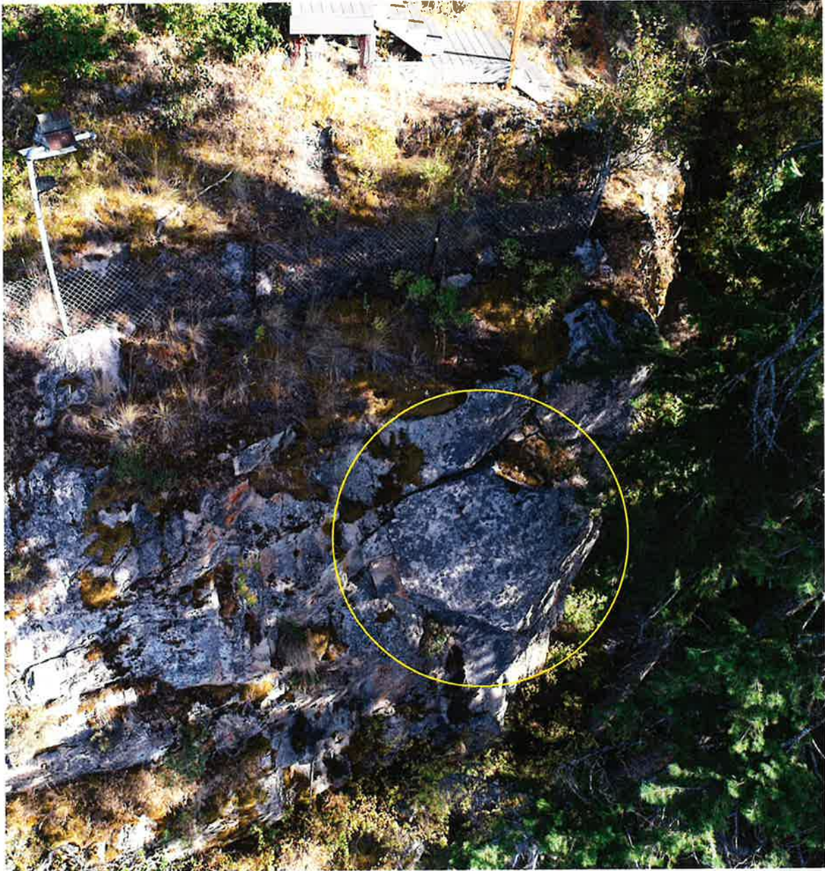
Figure 2. Loose rock block.
