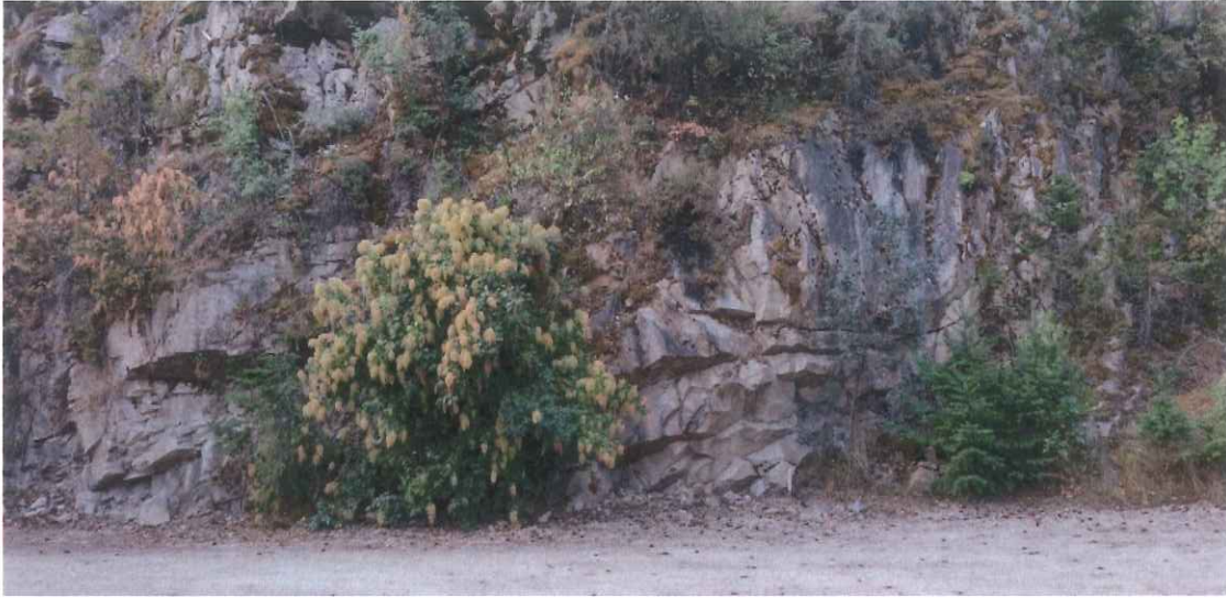
Photo 7- South sloped areas of property found to be undevelopable due to 10 m cliff facings.
