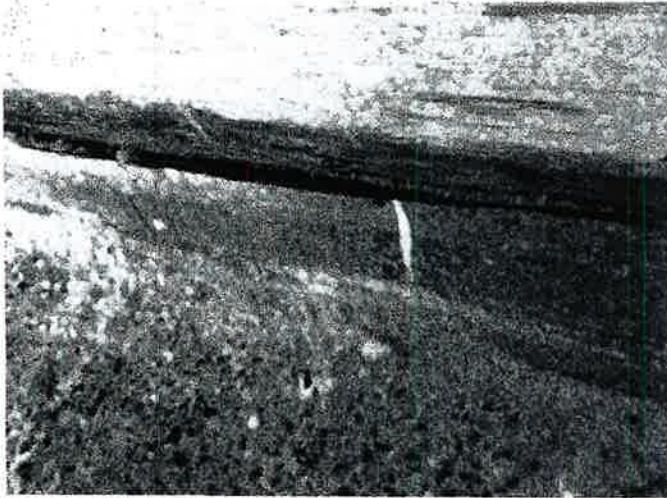
Flashing along back of sign and bare painted wood exposed
