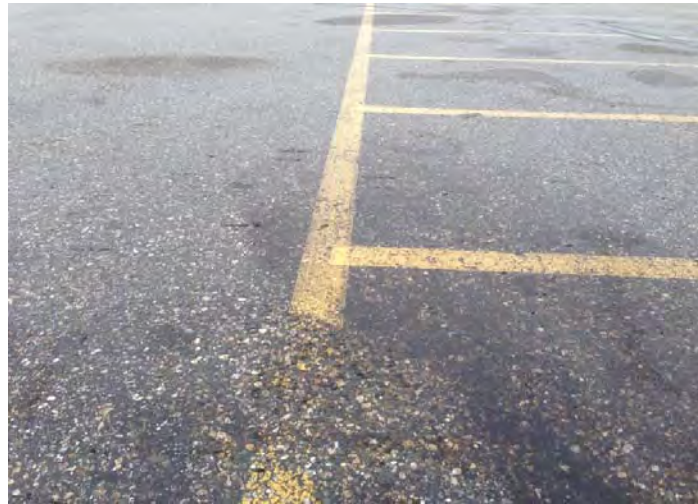
Photo 4:25 - Fuel spills near the fuel compound area in Apron #1
