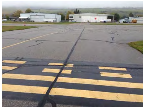
Photo 4:15 - Low Severity Cracking in Section 5
