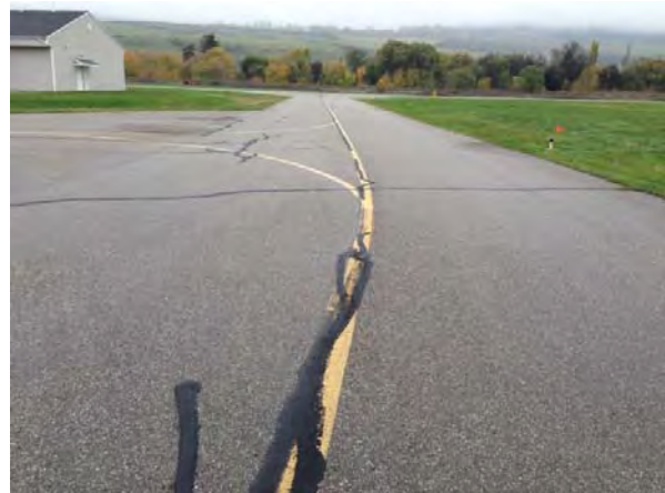
Photo 4:17 - Low Severity Cracking in Section 6
