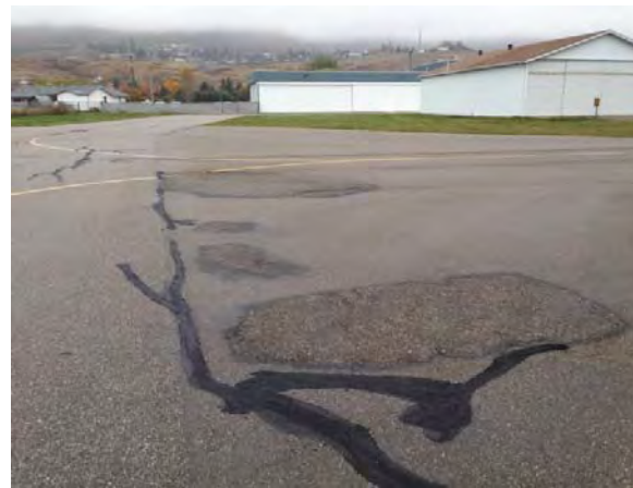
Photo 4:20 - Patches at intersection with Taxiway D
