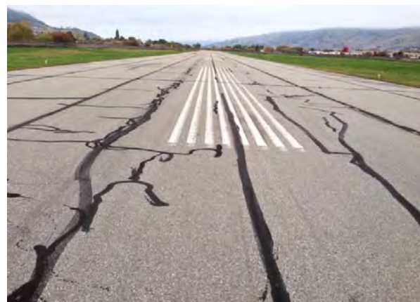
Photo 4:4 - Extreme extent of block cracking
