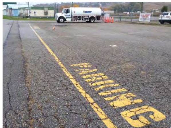
Photo 4:11 - Extreme Map Cracking in Section 4A
