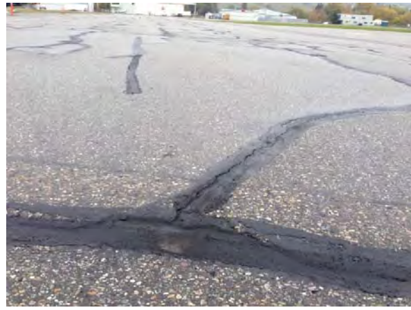
Photo 4:13 - High Severity Block Cracking in Section 4E
