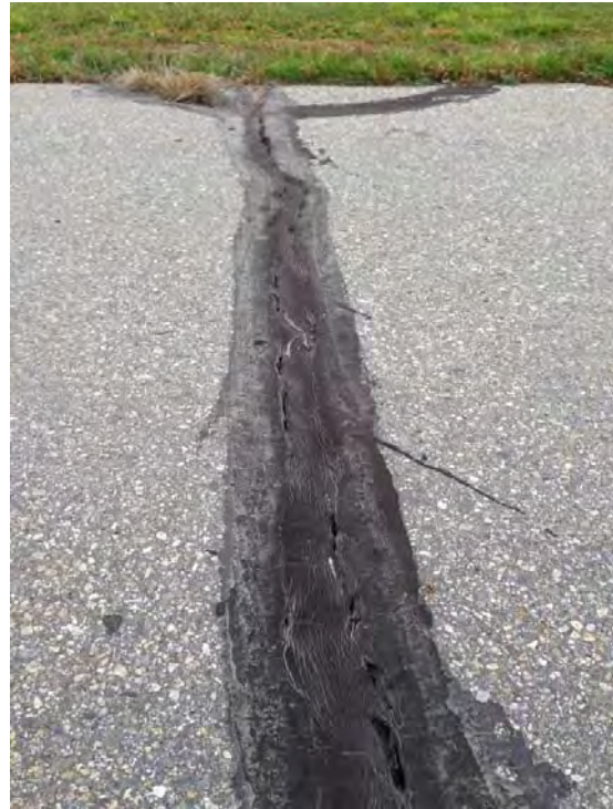
Photo 4:6 - High severity cracking
