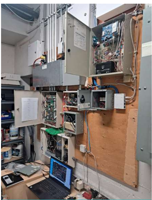
City Hall Climate Controls
