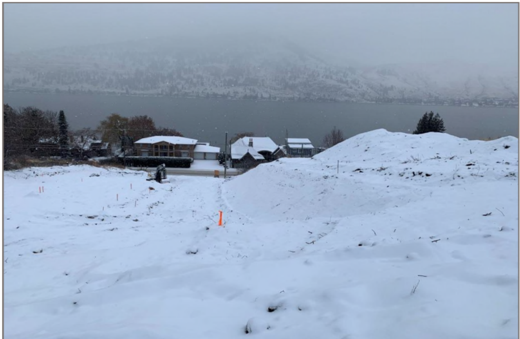
Photo 4: Project Site looking north along eastern property boundary (orange ribbon and stakes). Note: excavation extends beyond the eastern property limits.
