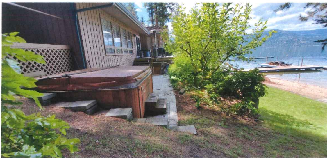
Photo 4: northeast corner of home, foundation here will require non-structural repair (refinishing) (May 2020).
