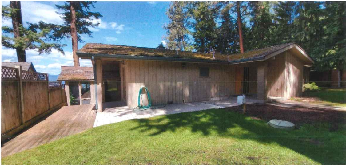
Photo 6: Southwest corner of home where foundation will require non-structural repair (refinishing). Looking north. (May 2020).
