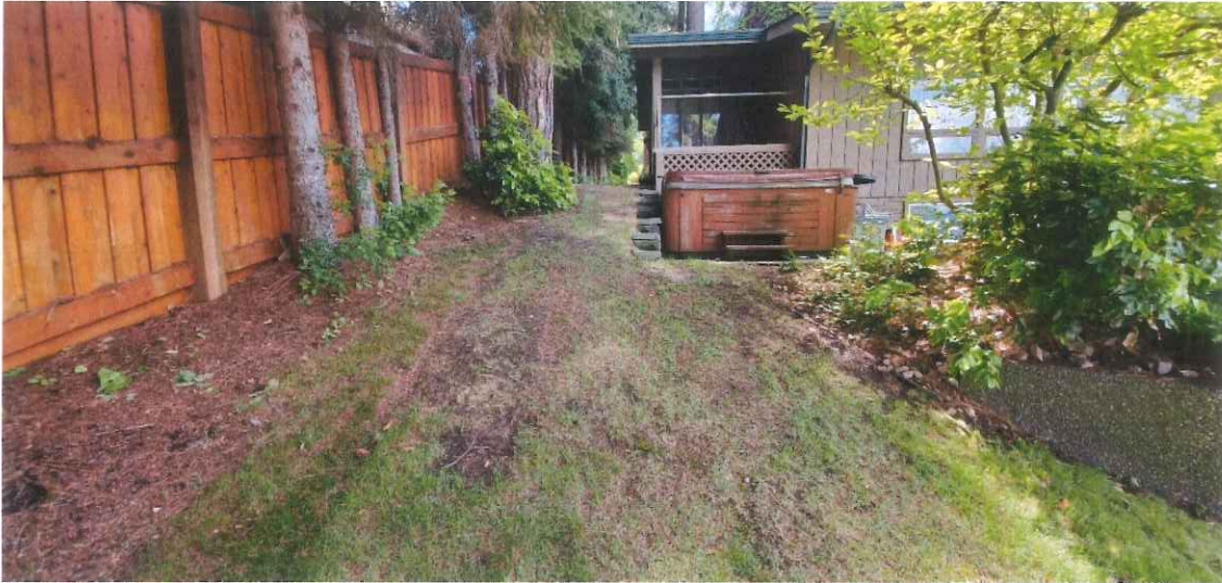
Photo 5: Looking south down the eastern property line. This corner of the home will require foundational repair (May 2020).
